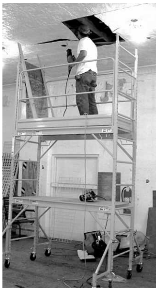
Chris Lantier of JD Contracting repairs the original tin ceiling at 7328 Carroll Avenue.
