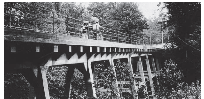
Built in 1909, the second bridge was a much more substantial structure that allowed Carroll Avenue to continue straight across Sligo Creek.
